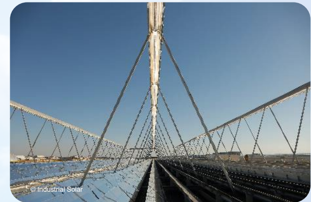
Fresnel (concentrated solar heat)
